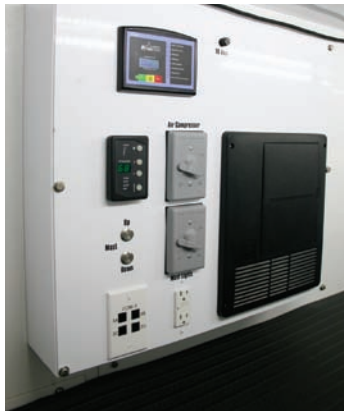
Central control of power generation, heating and cooling, mast tower, data ports and circuit breaker panel.
